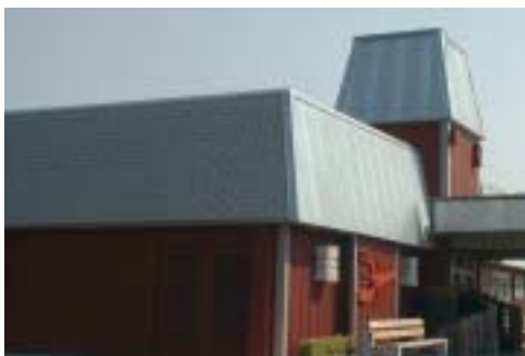
Unacceptable Hip on Deck Too Tall
