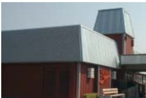
Unacceptable Hip on Deck Too Tall
